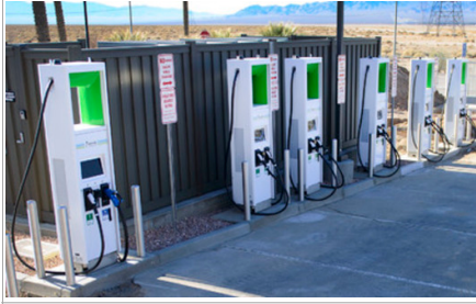
One of the state's newest electric-vehicle charging stations is located in Primm. (NV Energy)
