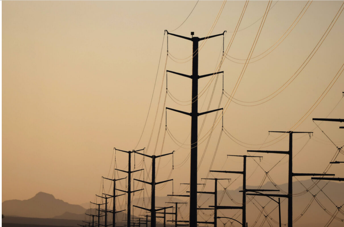
High-tension power lines over Moccasin Road in Las Vegas on Monday, July 17, 2023. (Jeff Scheid/The Nevada Independent)
